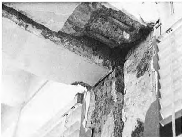
Fig. 56. Fracture of Girder-column Joint, Rear Interior, Municipal Building
