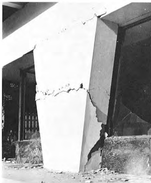
Fig. 61. Immeuble Paternelle, Detail of Column Fracture
