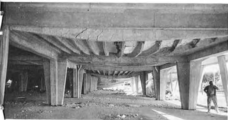
Fig. 66. Damage to Second Story Floor System of Market, Resulting from Collapse of Roof
