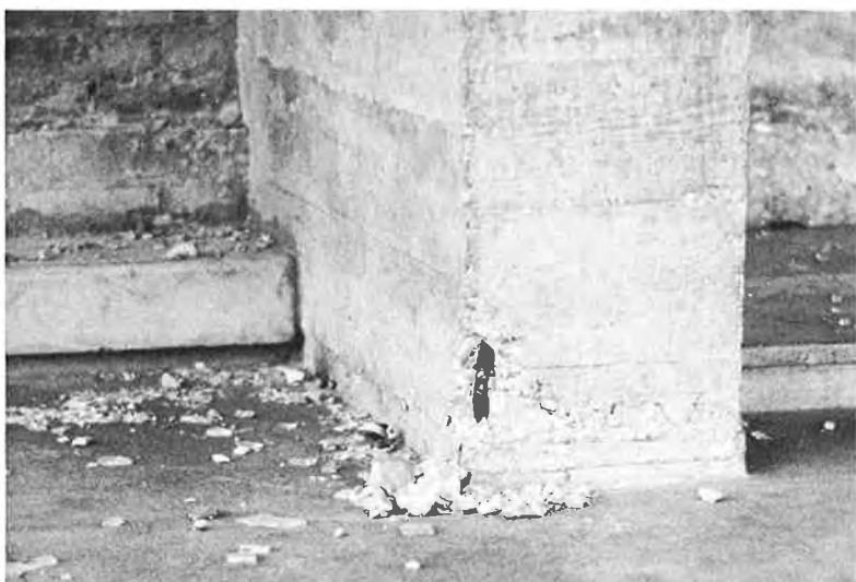
Fig. 59. Buckling of Reinforcement at Base of Column, Front Exterior of Municipal Building
