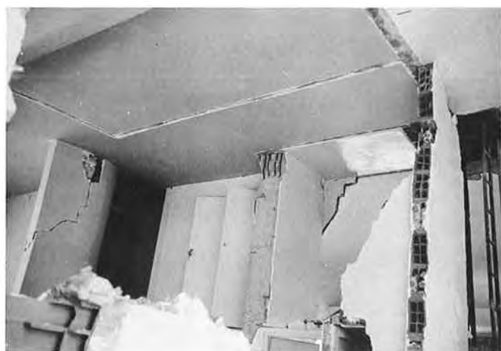
Fig. 63. Second Story Interior of Immeuble Paternelle, Showing Partition Damage
