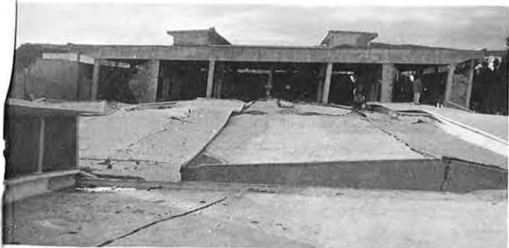
Fig. 65. Second Story of Market Building, Two Sections Collapsed, One Still Standing
