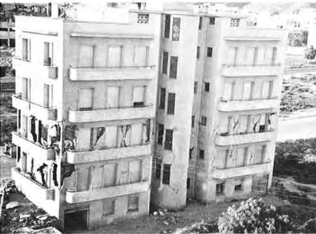
Fig. 69. Fracturing of Masonry Filler Walls Reveals Reinforced Concrete Frame
