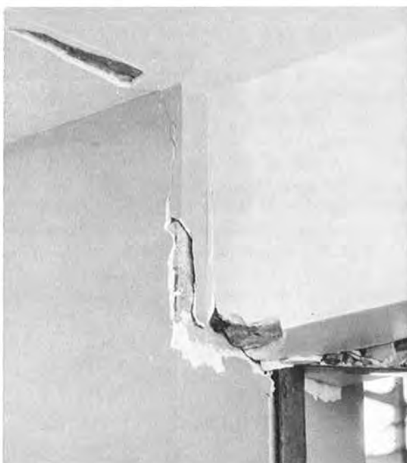
Fig. 58. Fracture of Joint at Interior Column, Municipal Building
