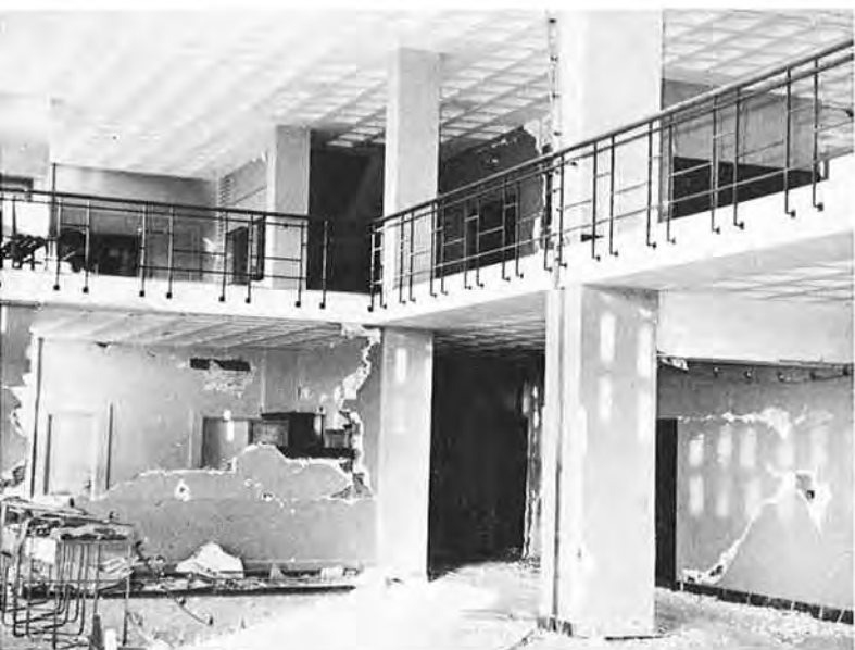
Fig. 54. Municipal Building, Damage to Tile Partitions
