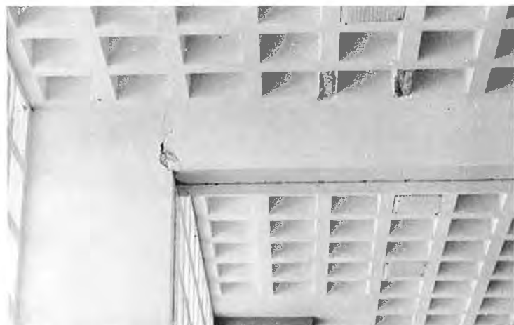
Fig. 55. Fracture of Girder-column Joint, Front Interior, Municipal Building
