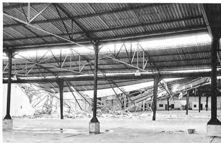
Fig. 90. Interior of Warehouse Crushed by Crane
