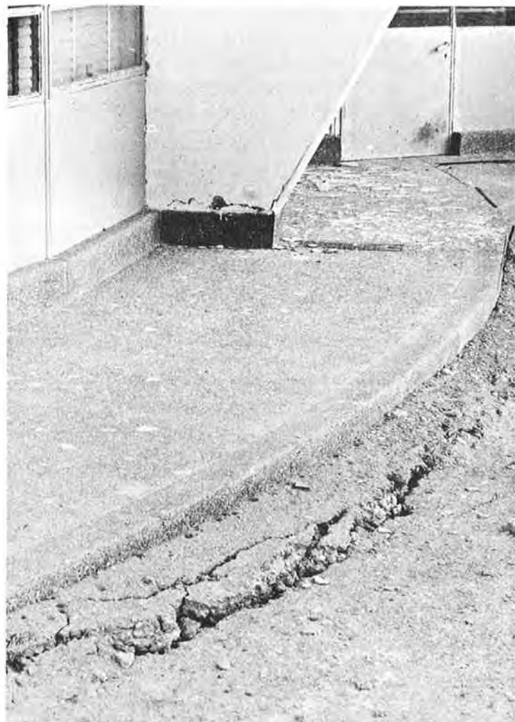
Fig. 78. Cracking at Base of Column of Customs House; Note Settlement of Soil With Respect to Structure
