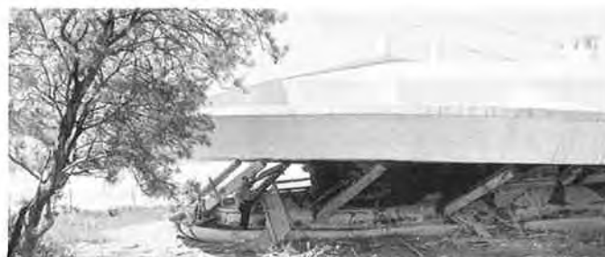
Fig. 74. General View of the Collapsed "La Reserve" Restaurant
