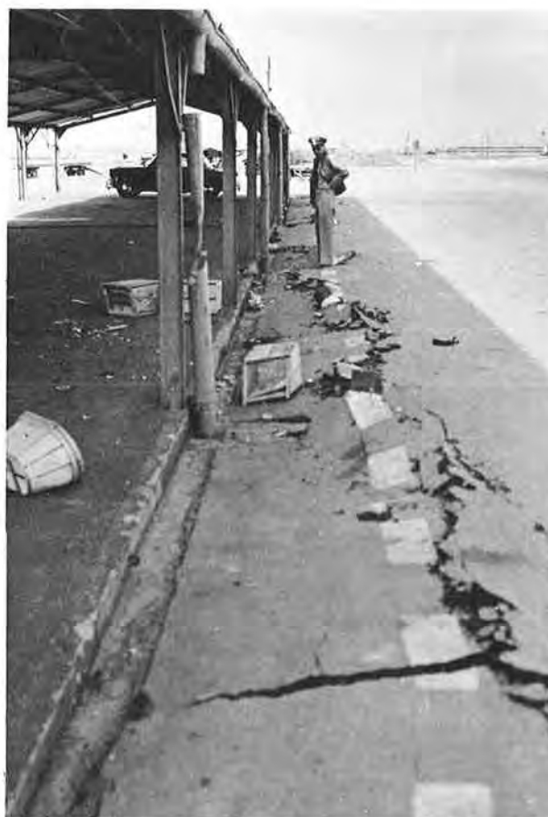
Fig. 91. Settlement of Steel Frame Shed Structure
