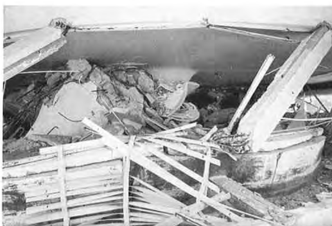
Fig. 75. Detail of the Collapse, Showing How Columns Have Punched Through the Floor System
